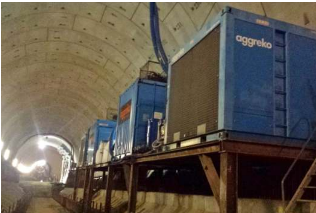
Two freezing units inside the main tunnel
