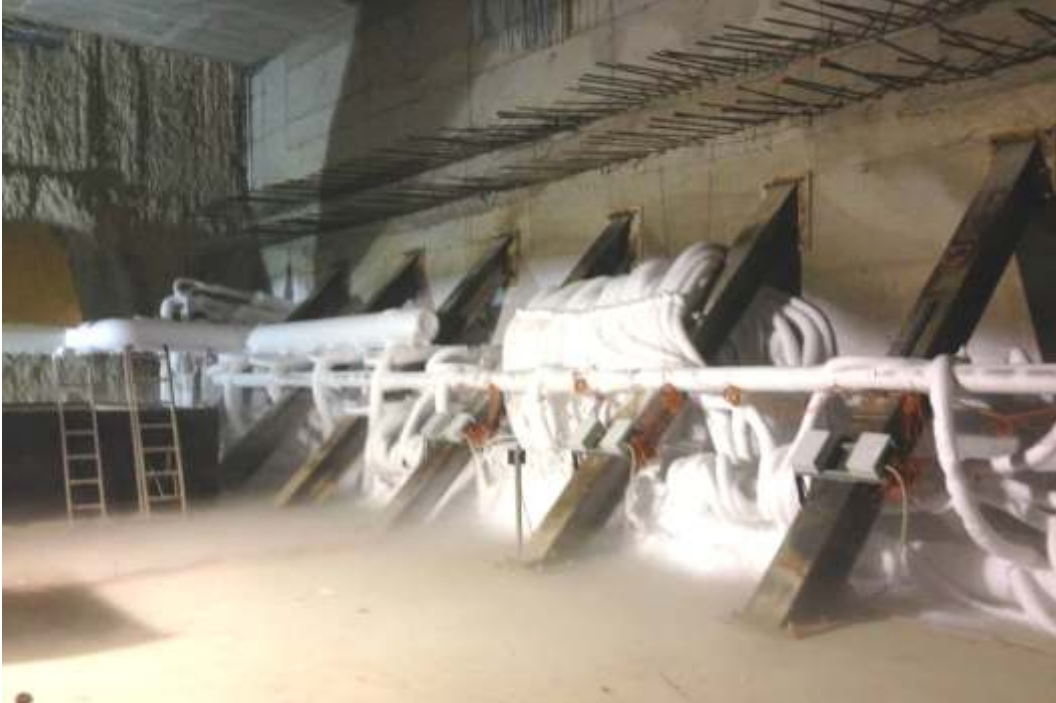
Liquid nitrogen installations - West Shaft
